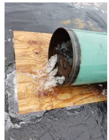
Effluent flow around 500 GPM
