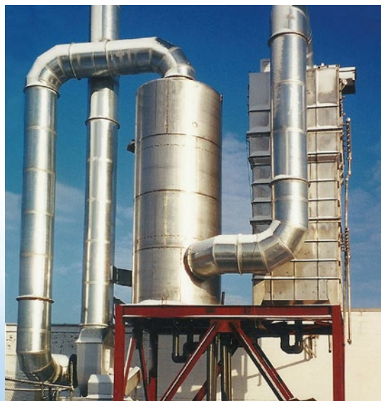
6,000 CFM Wet ESP and gas scrubber installation
