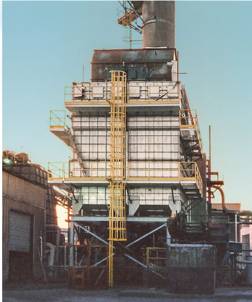
120,000 CFM Wet Electrostatic Precipitator treating waste fuel boiler emissions at a paper mill
