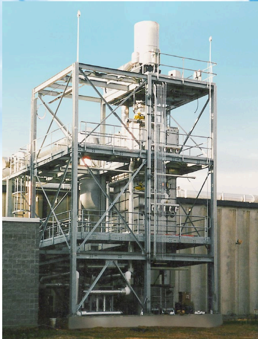
20,000 CFM Wet ESP for submicron particulate removal from oven exhaust at a textile plant
