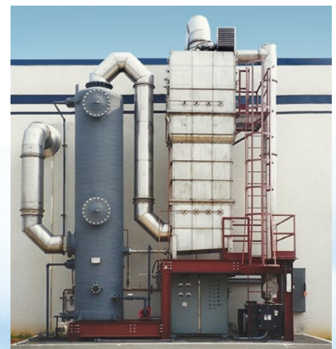
5,000 CFM Multi-Stage Scrubber System with FRP acid gas scrubber and 317SS Wet ESP
