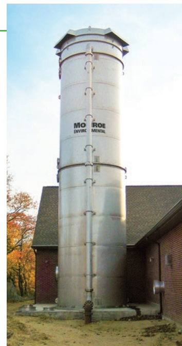
Air Strippers: Removes VOCs, ammonia, and other pollutants from contaminated water streams
