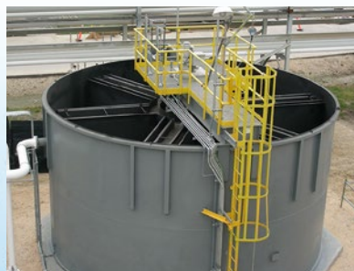
High rate Solids Contact Clarifier
