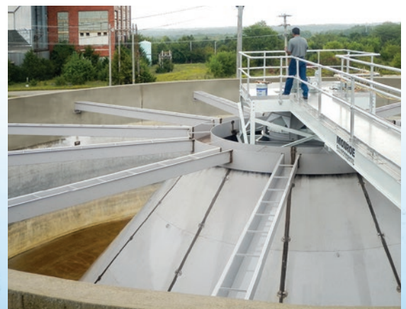
Solids Contact Circular Clarifier
