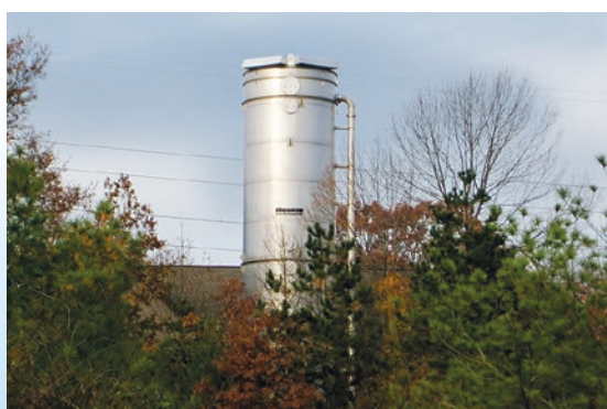
50 ft. x 13 ft. diameter stainless steel stripping tower for VOC removal at a potable water treatment plant
