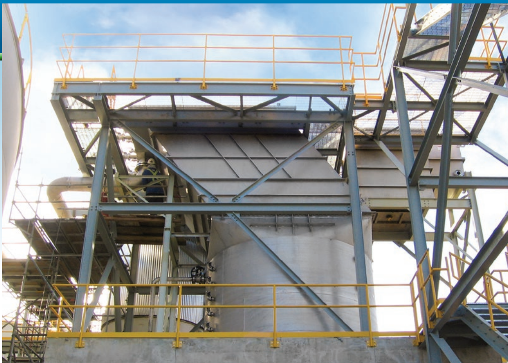
Vertical Plate Clarifier with thickener rated for 660 GPM
