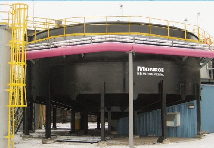
Left: 46 ft. diameter self-supporting Circular Thickener for separating blast furnace scrubber fines from wastewater at a steel processing plant
