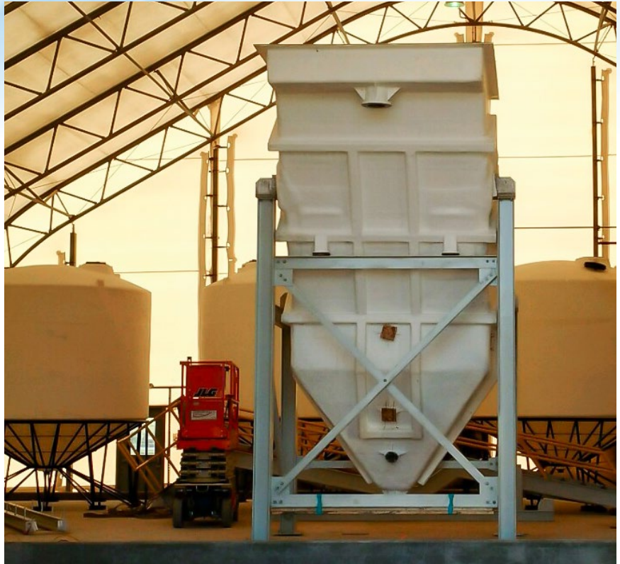
UV-resistant polypropylene modular laminar plate cartridges were recommended to help increase flow rate from 950 GPM to 1,350 GPM
