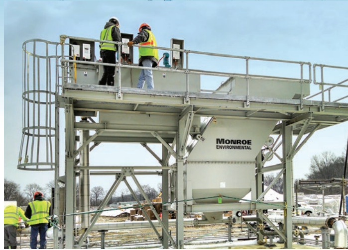
Installation of Vertical Clarifier for disc filter backwash with chemical mix tanks, access platform, ladder, and support structure
