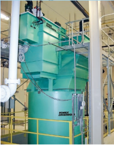
70 GPM Vertical Clarifier with flash and flocculation tanks, thickener, and FRP cover for landfill leachate treatment
