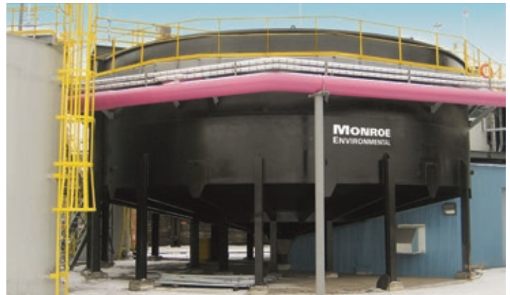
Circular Clarifier to remove TSS/fines from blast furnace scrubber wastewater. The 46 ft. diameter clarifier was elevated on legs for ease of access to sludge piping, and was designed to handle a 2,000 GPM max flow.
