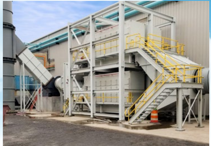
95,000 ACFM Monroe Multi-Stage Mist Collectors capture oil mist, PM, and fumes from rolling mill exhaust. The systems was capable of removing filterable and condensable PM with high-efficiency filters and a cooling coil/heat exchanger with chiller.
