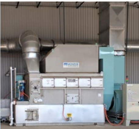
25,000 CFM Venturi Scrubber to capture and remove lubricant mist, particulate, and fumes from aluminum die casting operation. System included scrubber, fan, oil recovery unit, insulated liquid sump, and controls.
