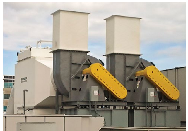
Dual-train exhaust ductwork with automated dampers and FRP fans provides maximum control over the scrubbing process.
