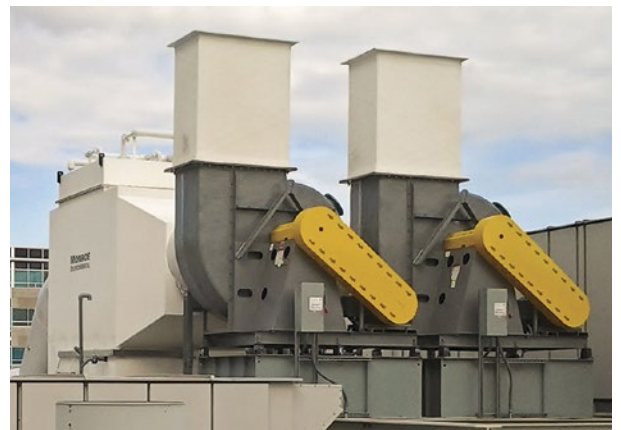
Dual-train exhaust ductwork with automated dampers and FRP fans provides maximum control over the scrubbing process.
