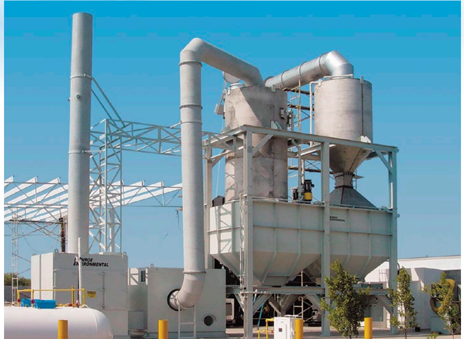
20,000 CFM Multi-Stage Scrubbing System for solid waste incineration process. (From right): Ceramic-lined inlet duct, rapid water quench, adjustable Venturi Scrubber, liquid clarification tanks, Packed Bed Scrubber, and Carbon Adsorber.
