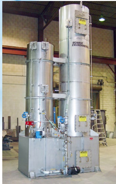
Vertical Quench Tower with Packed Bed Scrubber
