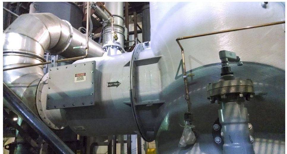
Inlet duct quench with horizontal spray configuration
