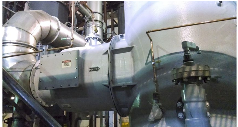
Inlet duct quench with horizontal spray configuration
