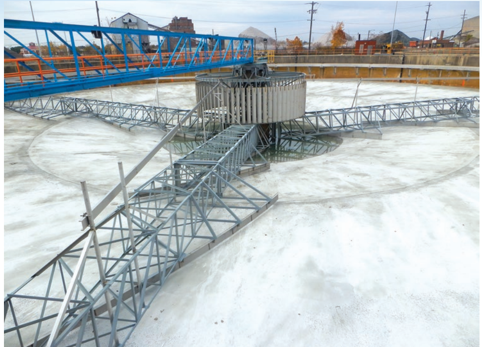
Rebuilt Circular Clarifier with higher efficiency spiral scrapers
