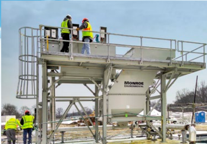
150 GPM Vertical Plate Clarifier to treat disc filter backwash at natural gas power station. System included clarifier, chemical mix tanks, access platform, ladder, and support structure.
