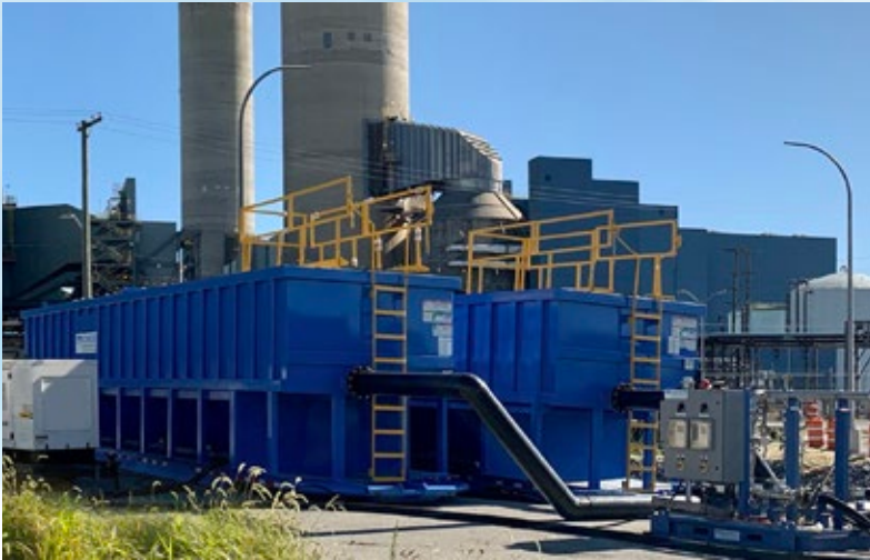
Monroe X-Flo Mobile Clarifiers™ treating fly ash from wash down water at a coal-fired power plant during a planned outage. Clarifiers treated up to 2,000 GPM and included sludge underflow pumps.
