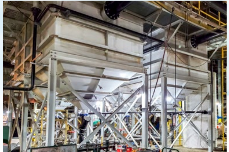
Two Horizontal Clarifiers for solids and oil removal from stormwater at a coal-fired power plant. Scope included clarifiers with bolted steel covers, flocculation tank with mixer, skimmed oil storage tanks, and access platform. Clarifiers were rated for 600 GPM each.
