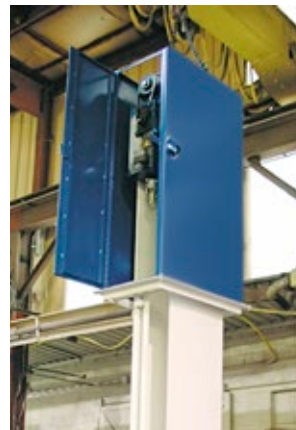
Monroe belt skimmer Oil Recovery Unit for oil removal from wastewater holding basin at a large coal-fired power plant. The belt retrieved oil from tanks approx. 20 ft. below the mounting surface.
