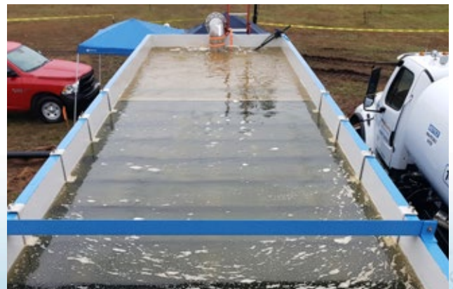
Monroe X-Flo Mobile Clarifier™ for continuous treatment of hydrotest water during commissioning of a new gas pipeline. Treated flow varied between 500 – 1,000 GPM.
