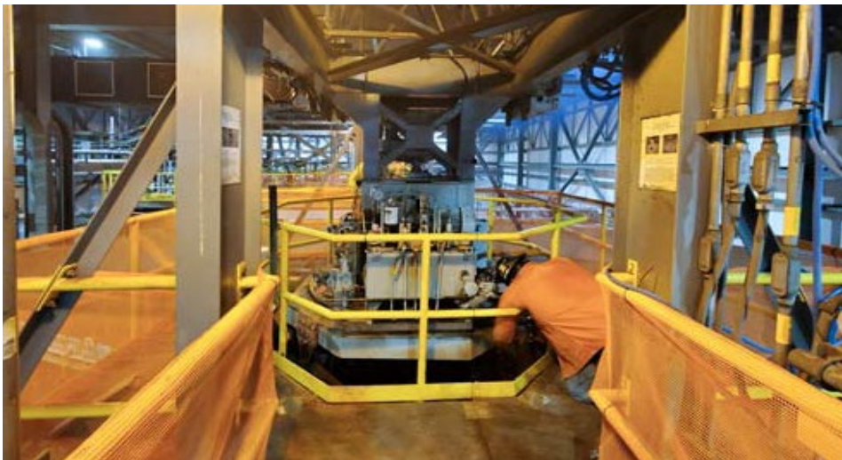
Clarifier drive rebuild for FGD recycle clarifiers at a power plant. The solids contact clarifier drives (non-Monroe unit) were misaligned and wearing rapidly. The drive rebuild prevented a possible emergency shutdown if they had failed.
