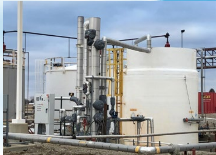
200 ACFM Packed Bed Scrubber for removal of HCl fumes from acid storage tank at biodiesel plant. Unit was insulated and heated for freeze protection.
