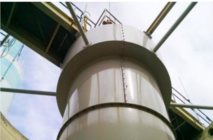
32 ft. diameter Solids Contact Clarifier treating river water for government energy plant. The clarifier included reaction well, mixer, sludge rakes, drive, launders, and access bridge.
