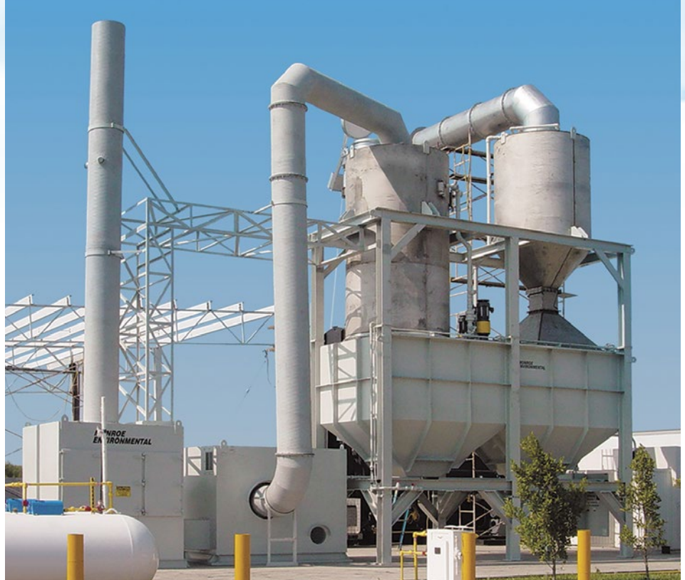
20,000 CFM Multi-Stage Scrubbing System for solid waste incineration process. (From right): Ceramic-lined inlet duct, rapid water quench, adjustable Venturi Scrubber, liquid clarification tanks, Packed Bed Scrubber, and Carbon Adsorber.
