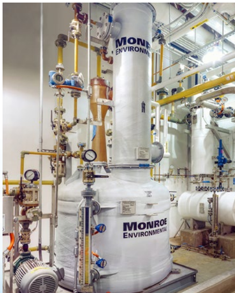
Two-stage wet scrubbing system with eductor venturi and packed tower for HCl and SO 2 reduction from pharmaceutical manufacturing process exhaust
