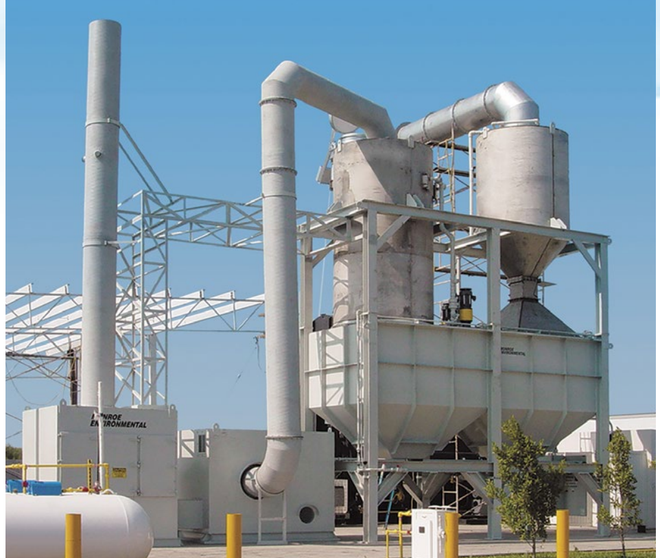
20,000 CFM Multi-Stage Scrubbing System for solid waste incineration process. (From right): Ceramic-lined inlet duct, rapid water quench, adjustable Venturi Scrubber, liquid clarification tanks, Packed Bed Scrubber, and Carbon Adsorber.
