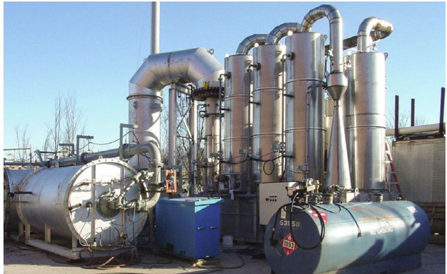
Below: Multi-Stage Scrubbing system with inlet quench, 3-stage Packed Bed Scrubber, high energy Venturi Scrubber, liquid chiller/condenser, gas reheater, PAC injection system, baghouse, and Carbon Adsorber for toxic gas incineration
