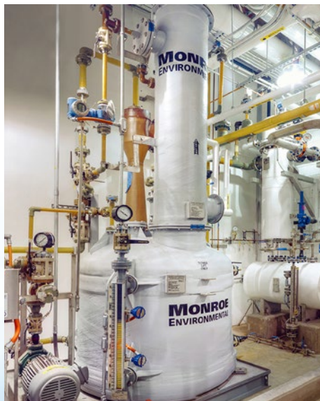
Two-stage wet scrubbing system with eductor venturi and packed tower for HCl and SO 2 reduction from pharmaceutical manufacturing process exhaust
