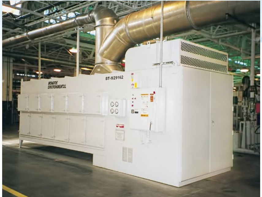
18,000 CFM Spiral Tube Mist Collector at an automotive engine assembly plant
