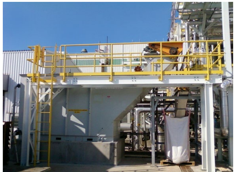
150 GPM Horizontal Clarifier with drag conveyor
