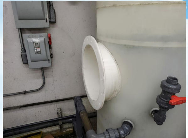
A new additional access door was added to allow for future cleaning/improved maintenance.
