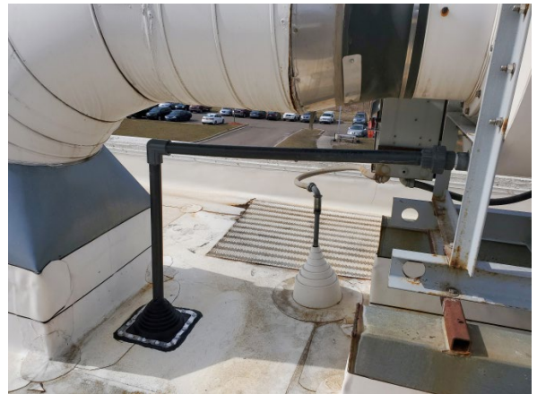
Drain lines from the fan were installed, allowing a path for acid to drain back into the scrubber.
