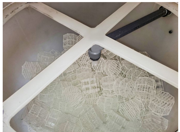
Improved packing media, mist pads, and new spray nozzles were installed to resist build-up of bacteria and particulate.
