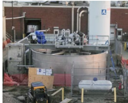
350 GPM Circular Clarifier with enhanced custom skimming system to handle foam and starch accumulation in wastewater for a snack foods company.
