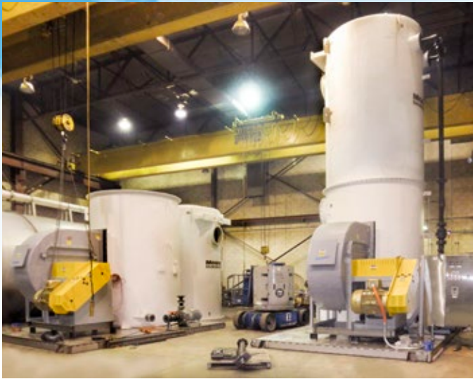
Liming drum exhaust scrubbing – H 2 S neutralization and fume control at a leather tannery. Dual 20,000 ACFM Packed Tower Scrubbers, FRP construction, with fans, pumps, and controls.
