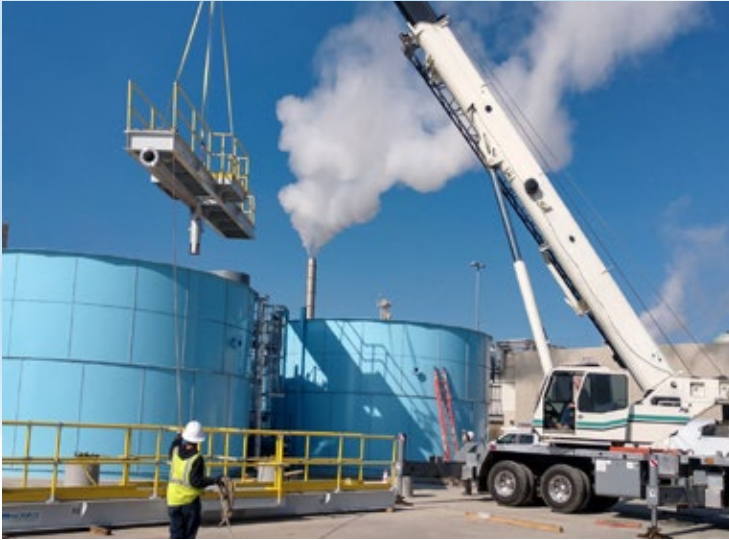
Two Primary Clarifiers capable of processing 1.25 million gallons per day with a custom designed enhanced skimming system to remove FOG in wastewater for a snack production plant.
