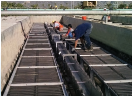
Plate Settler for enhanced separation of solids in a wastewater digester at a brewery. The plates were constructed from 304SS and have 120 modules.
