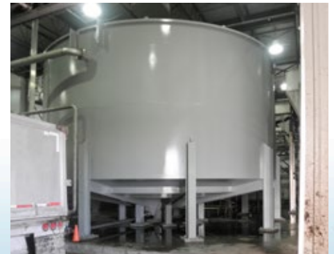
30 ft. diameter, 600 GPM Circular Clarifier with integral leg set for potato wash process at french-fry production facility.
