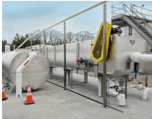
API Oil/Water Separator for oil removal for snack chip production facility wastewater with oil recovery/ concentrating tank and waste oil storage tank. The system was selected to enhance the plant's FOG removal capabilities.
