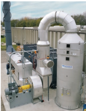
Monroe Multi-Stage Scrubbing System with Venturi Scrubber and Cyclonic Separator to remove particulate from food dryer exhaust prior to VOC destruction with a regenerative thermal oxidizer.
