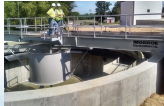
Circular Clarifier rebuild for wastewater treatment at a soft drink bottling facility. The internal mechanism, bridge, and drive were replaced in the 42 ft. diameter unit.
