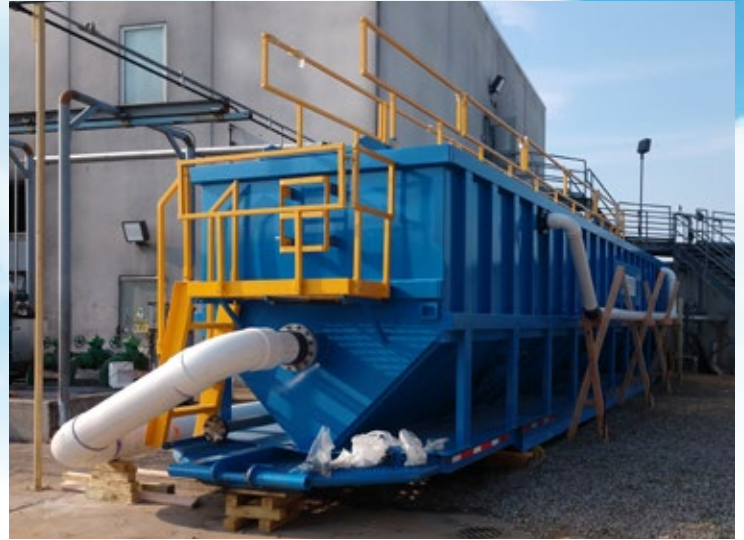
Rental X-Flo Mobile Clarifier™ with sludge removal pumps to bypass 40 ft. diameter secondary clarifier during rehabilitation at a snack chip plant. The X-Flo produced better effluent during temporary treatment than the existing clarifier during normal operation!
