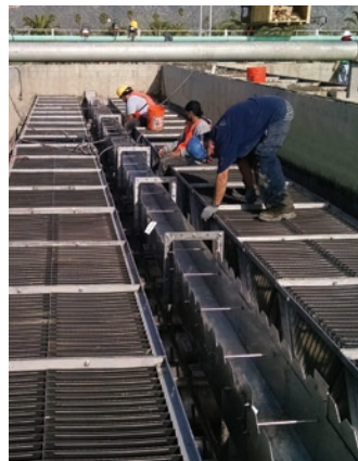
Plate Settler for enhanced separation of solids in a wastewater digester at a brewery. The unit was constructed from 304 SS and has 120 modules.
