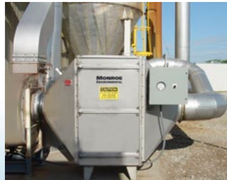
10,000 CFM horizontal flow, multiple tray Carbon Adsorber for odor control at a grainary.
