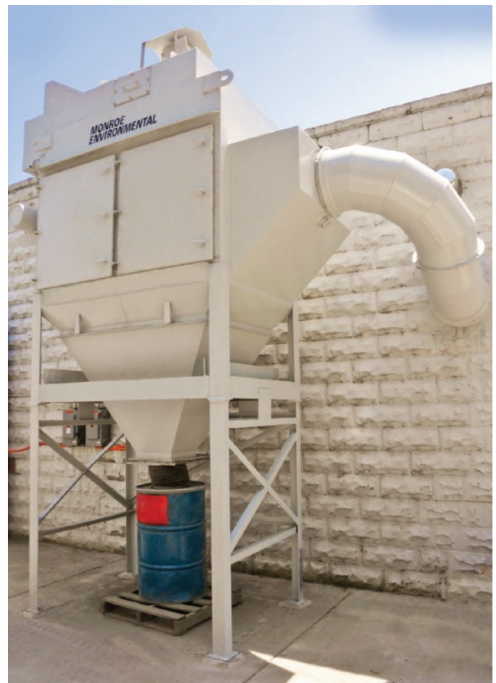
Dust Collector for sandblasting and painting operation
