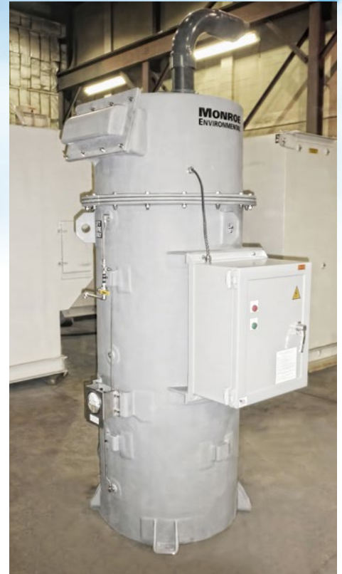
200 CFM Carbon Adsorber, FRP construction, with control panel for H 2 S removal at a municipal lift station
