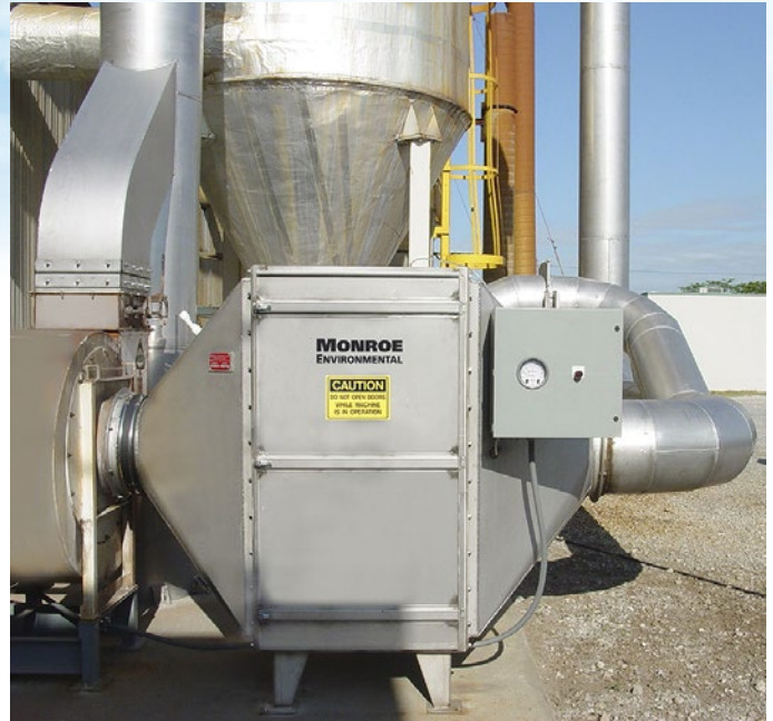
10,000 CFM Carbon Adsorber to filter the air stream and remove the foul odors
