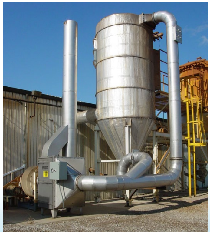
Carbon Adsorber with interconnecting ductwork and a discharge stack
