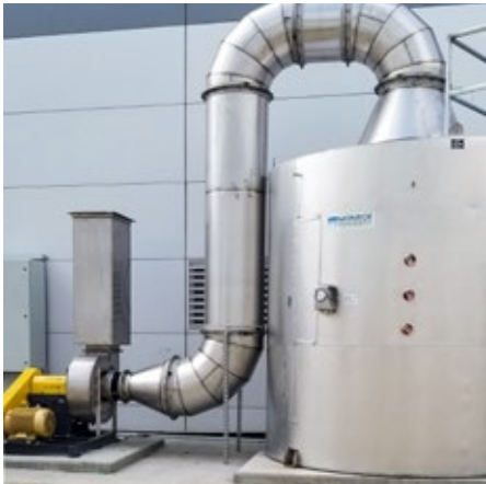
4,500 CFM Carbon Adsorber for an automotive battery manufacturer's VOC abatement system to exhaust ozone and other organic compounds harmful to workers from a manufacturing clean room.
