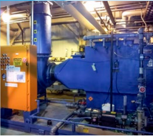
2,500 ACFM Packed Bed Scrubber with fan and controls to remove H 2 S fumes from acid cracking tanks at an axle manufacturing plant. Scrubber is constructed from FRP and has been operating for nearly 30 years.
