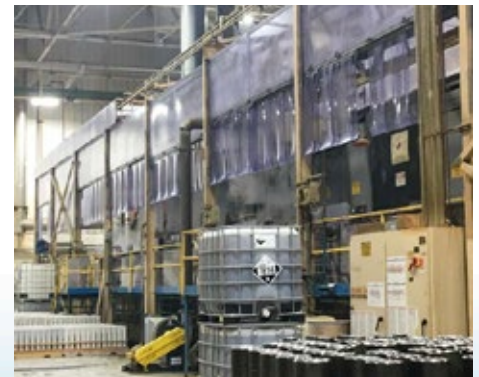
Modifications to existing coating line operations saved auto parts supplier $600,000 and solved acid mist and ventilation problems.
