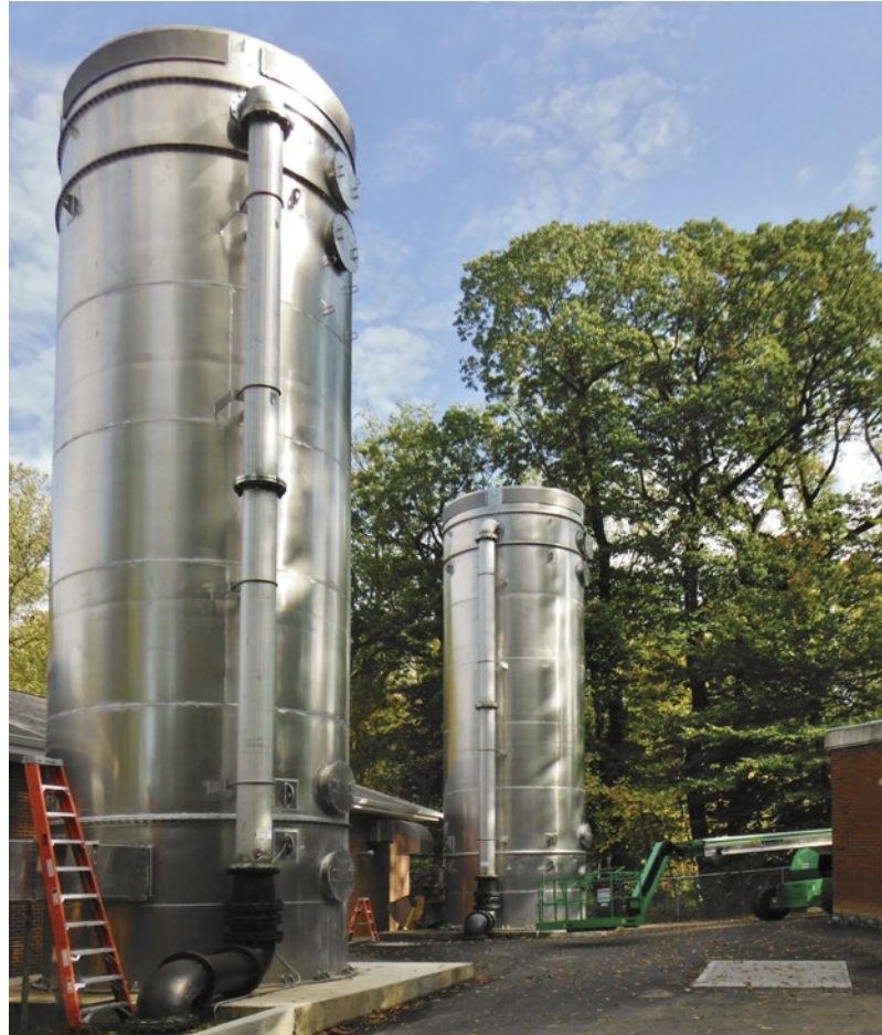
Air Stripping Towers installed at a water treatment plant
