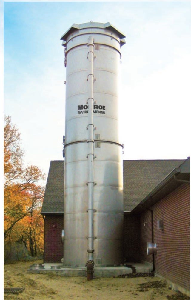
Air Stripper for VOC removal – Monroe's engineered unique air discharge arrangement reduces the noise allowing for quieter operation.
