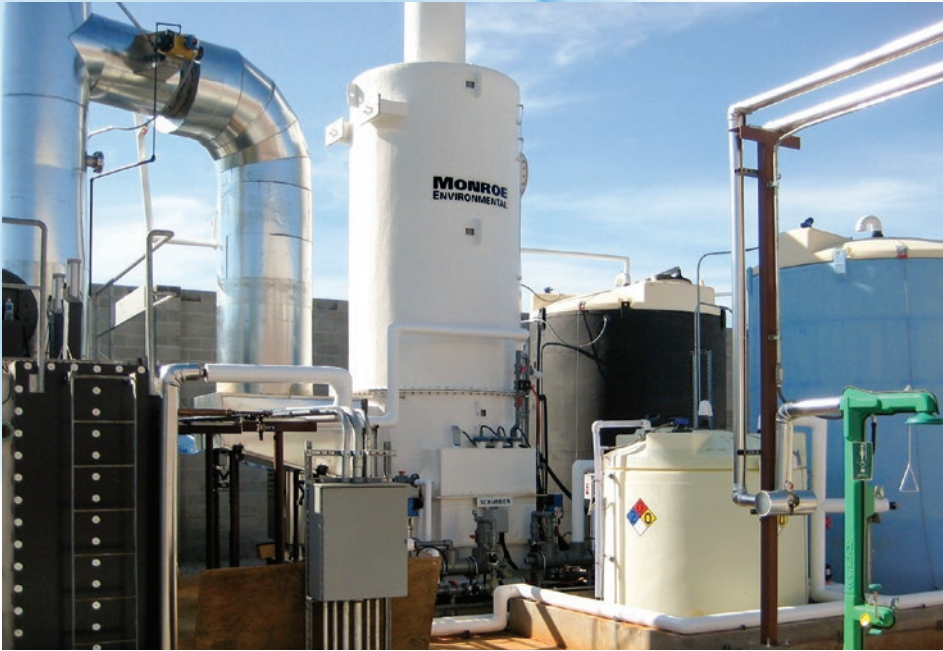
12,500 CFM scrubbing system for HCl and Cl 2 removal from RTO exhaust
