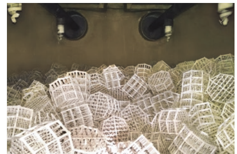
Non-plugging spray nozzles above bed of loose fill polypropylene packing
