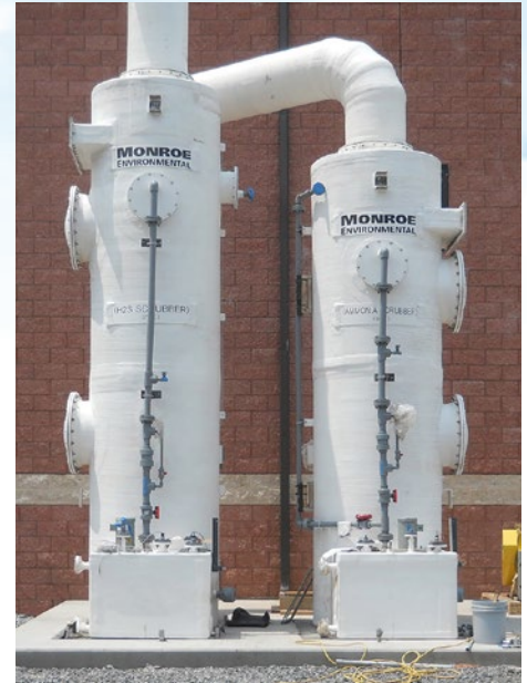
Two-stage Packed Bed Scrubber to remove acids and alkalis from dryer exhaust gas
