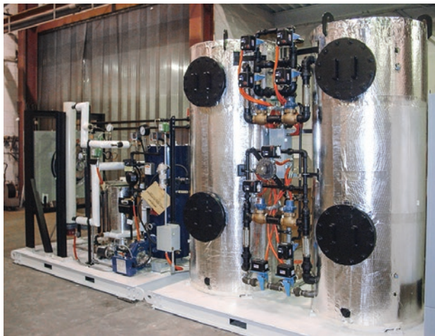
High pressure scrubbing system to remove sulphur compounds from a propane gas supply
