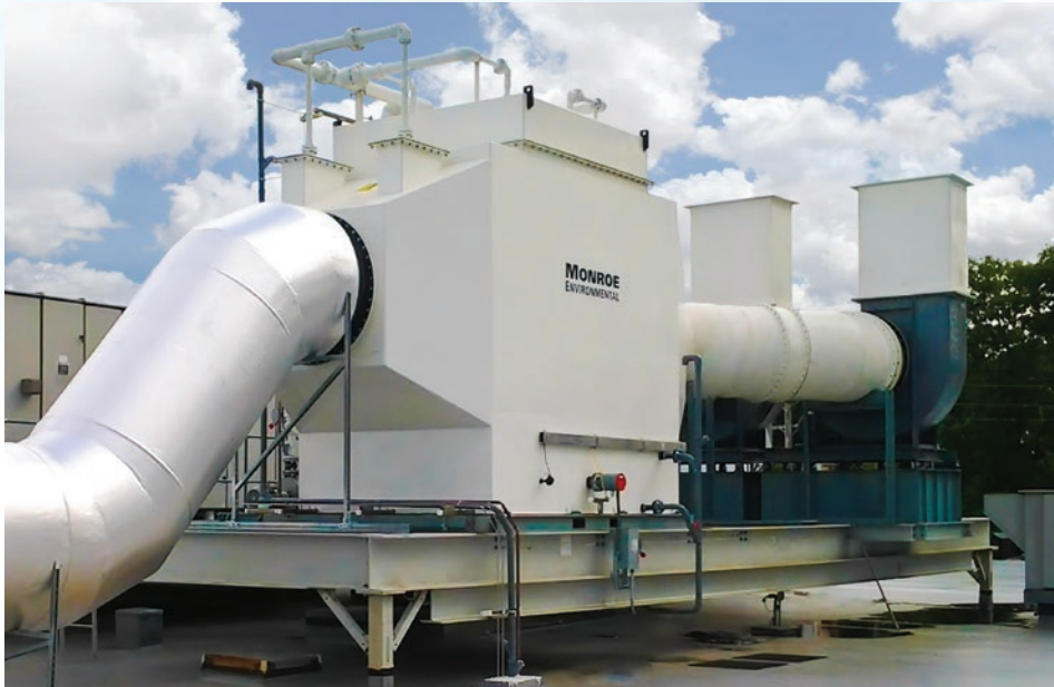
30,000 CFM Horizontal Packed Bed Scrubber with polypropylene construction to remove chemical fumes emitted from acid-dip tanks at a semiconductor manufacturing facility. Dual-train exhaust ductwork with automated dampers and FRP fans provides maximum control over the scrubbing process.
