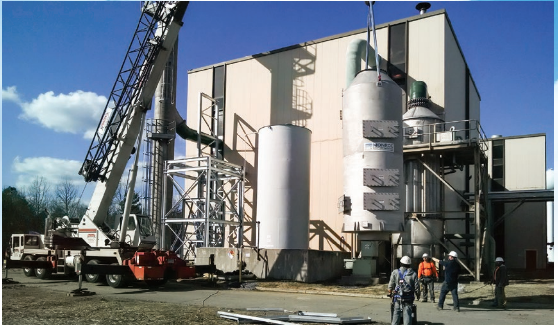
Packed Tower Scrubber for SO 2 removal from waste incinerator exhaust, 316 SS construction
