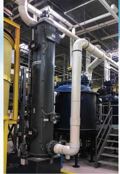
Fume Scrubbing: 1,200 CFM Packed Tower Scrubber; PVC construction with top-mounted fan for removal of iodine fumes from reactor tanks
